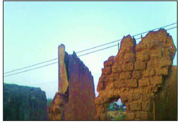
Plate 4: Erosion of Brick Mortar Joint
