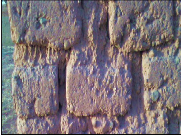
Plate 1: Partial Collapse of Mud Building
