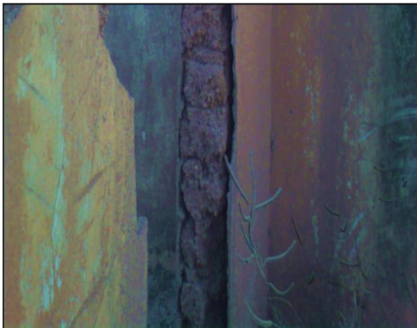
Plate 2: Crack at the Corner of Earthen Wall
