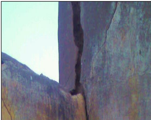
Plate 3: Flaking Due to Water Infiltration
