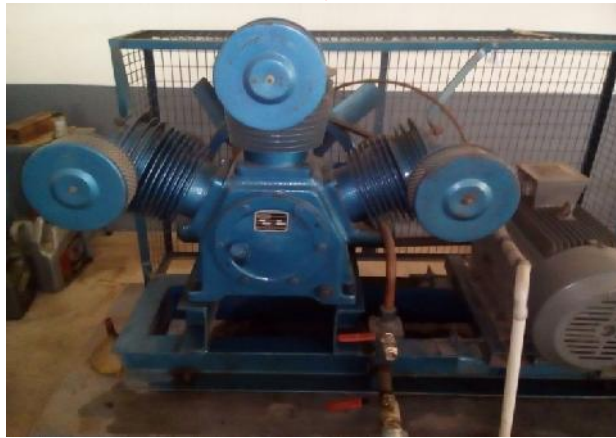
Figure- 5.4 Air Compressor
